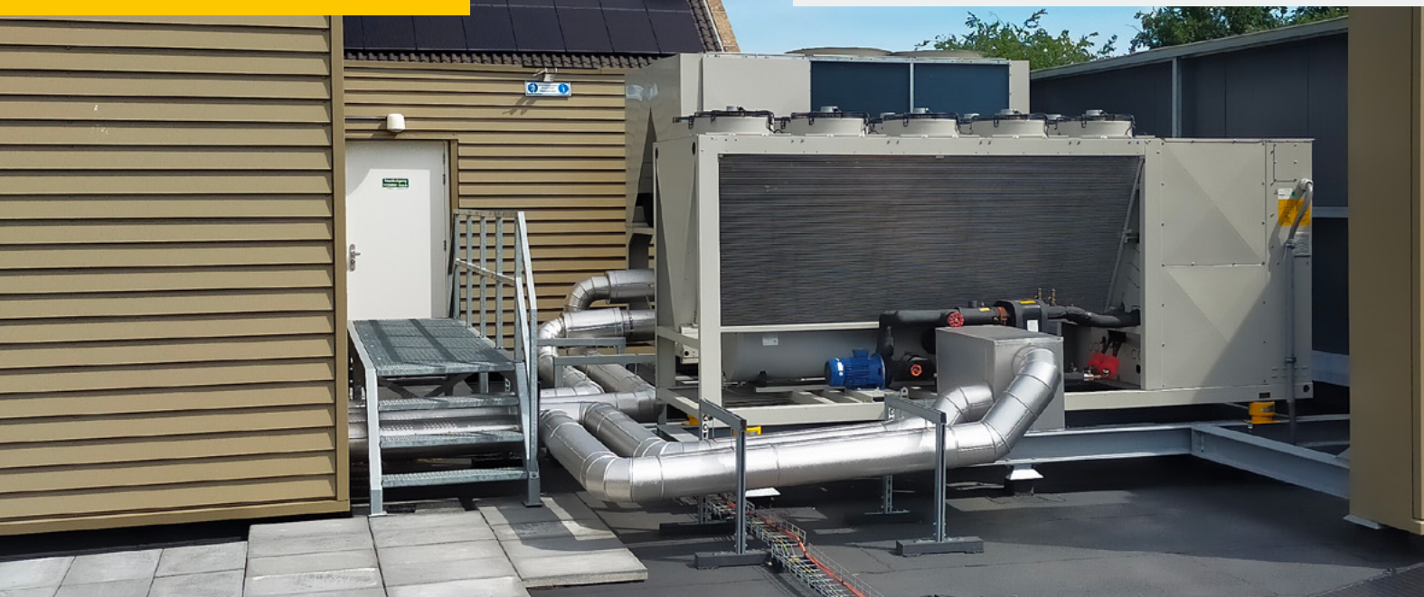
Vibration Isolation of Heat Pumps on Residential Building Waalwijk, Netherlands
